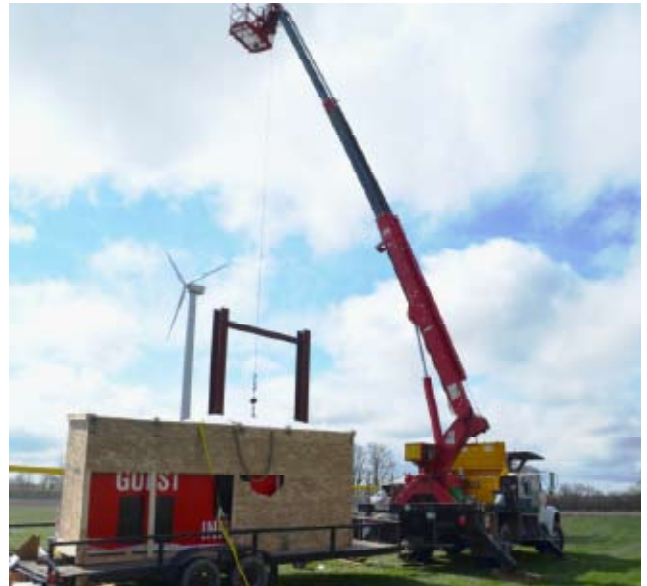
Brady Signs prepares the score board for its ascent high atop the twin I-beam stanchions.
